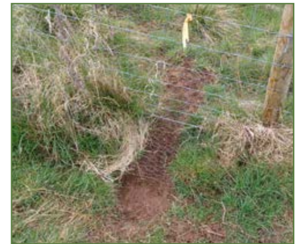
Regular fence checks are required to identify such as this breach caused by badgers
